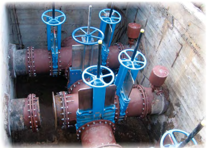
Sewage water treatment application
