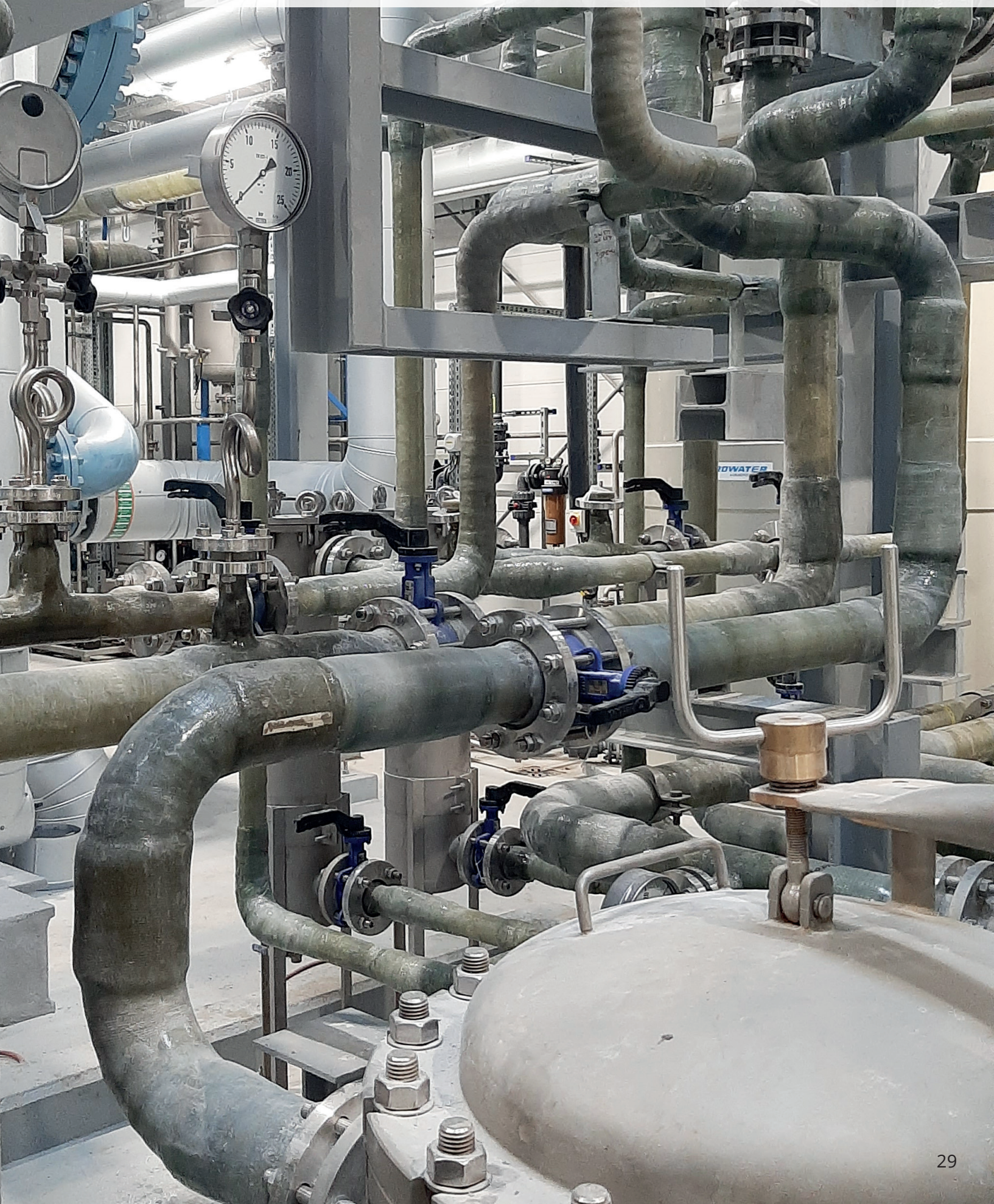
Geothermal-biomass heat plant, PN16, 2023
