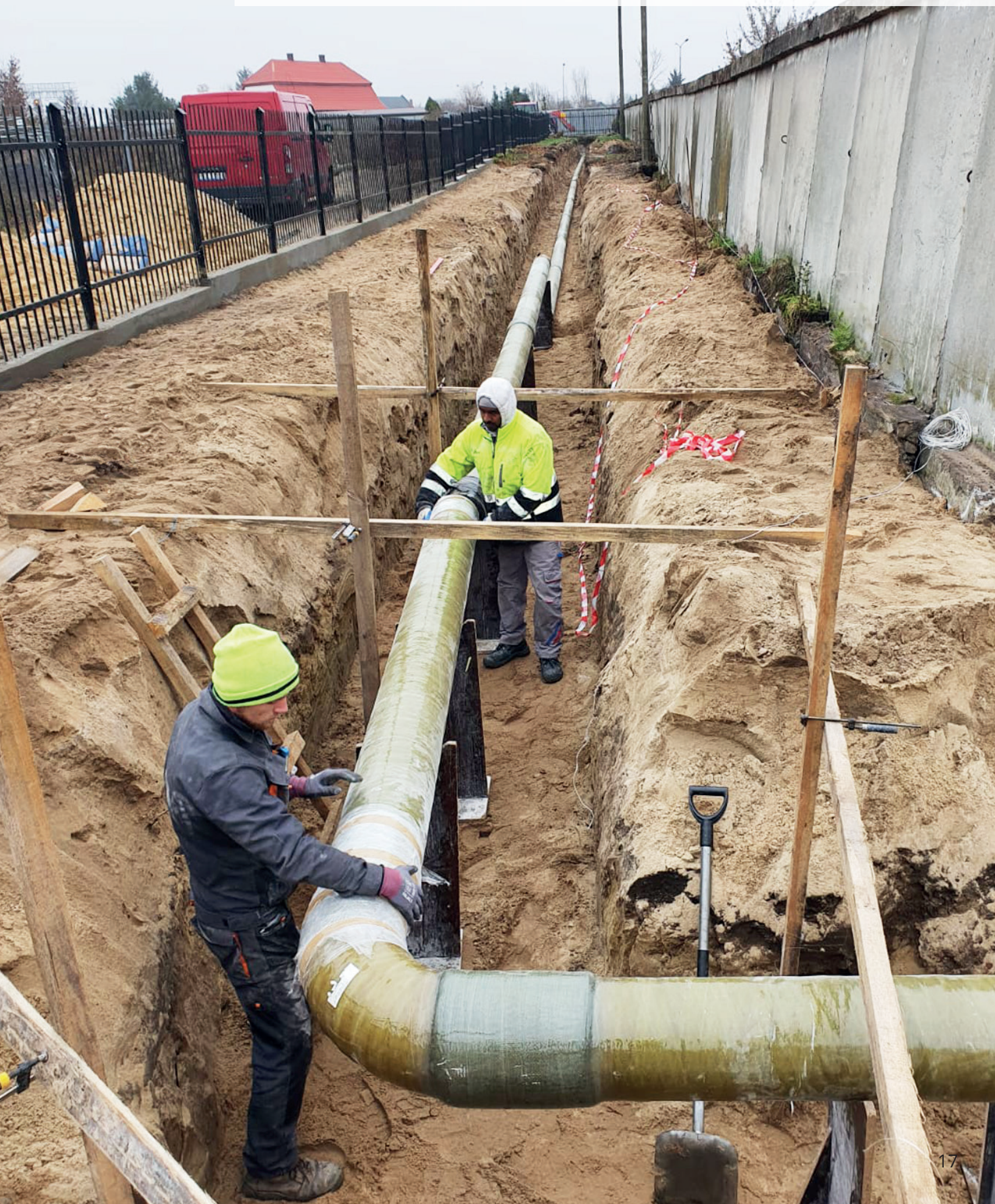
Geothermal heat plant PN16, 2022-2023
