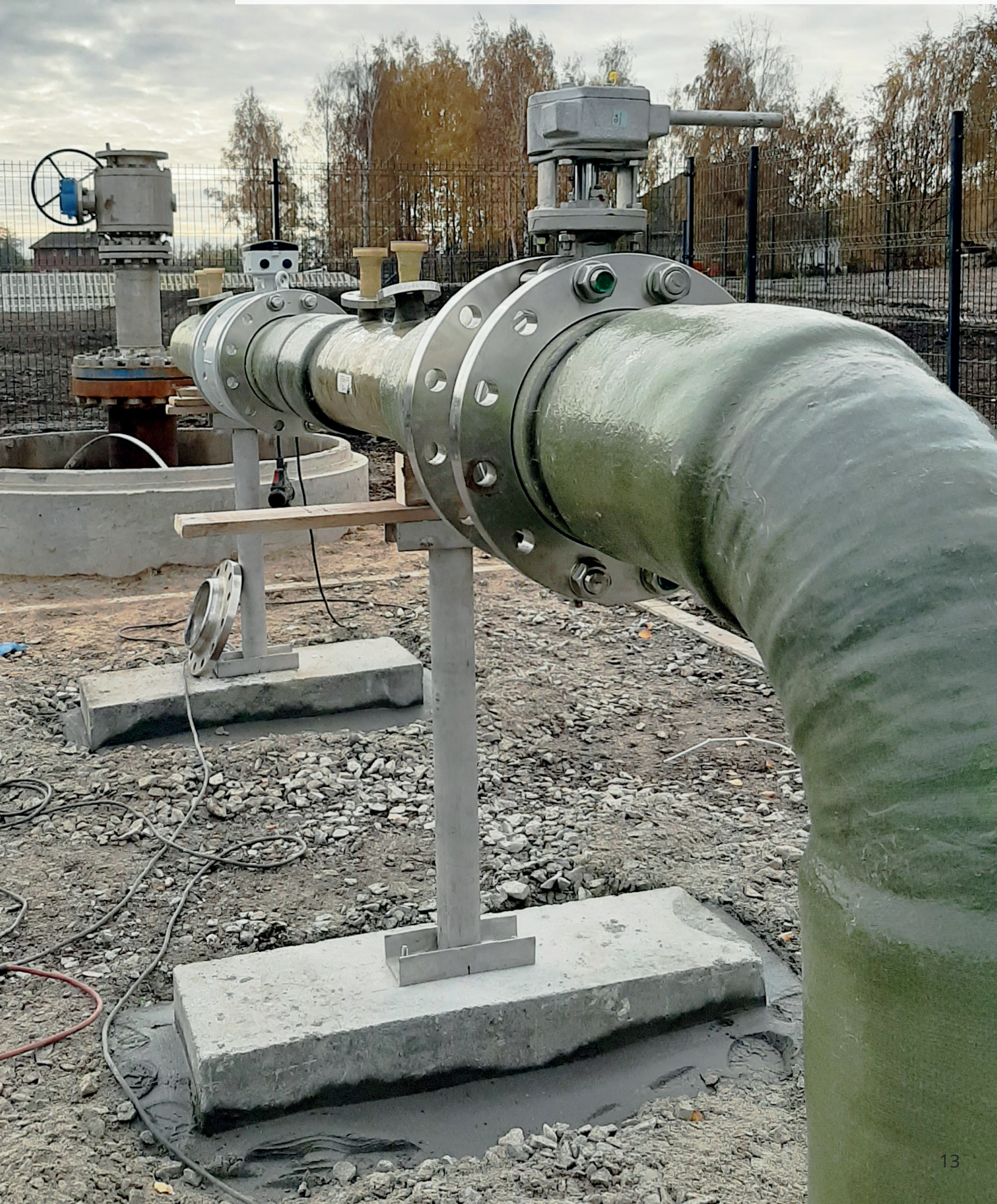
Geothermal-biomass heat plant PN16, 2023
